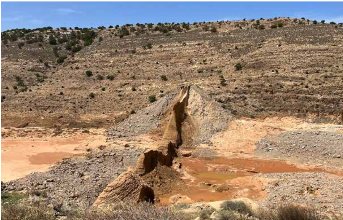
What remains of the Wadi Bu Mansur dam, 13km south of Derna in eastern Libya days after floods caused its collapse, September 2023.
